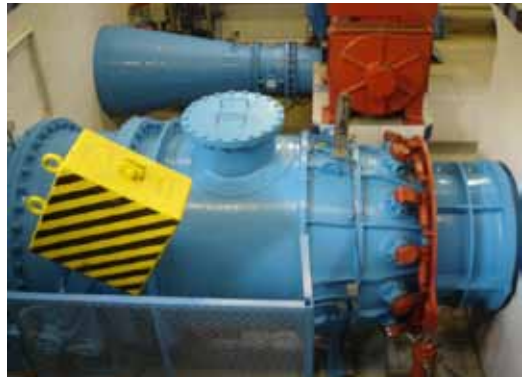
Hydropower installation Prad.
